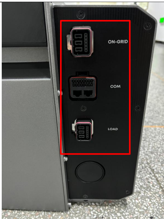
Detail view of AC grid connector, backup connector, and communication ports.
